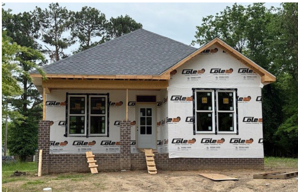
1314 Oscar Cross under construction with the help of the New Construction Grant
